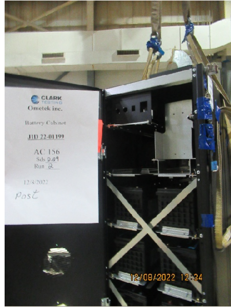
Figure 28: Run 2 Post-Test Condition
