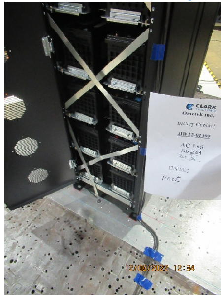
Figure 29: Run 2 Post-Test Condition
