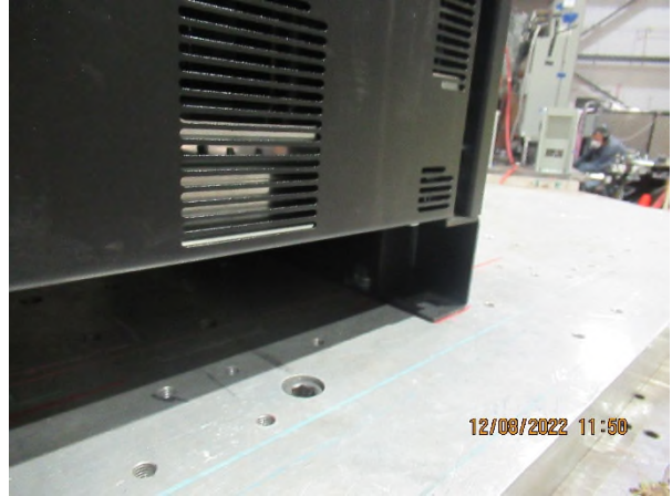
Figure 17: Run 1 Post-Test Condition
