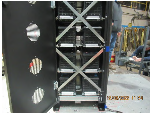
Figure 20: Run 1 Post-Test Condition
